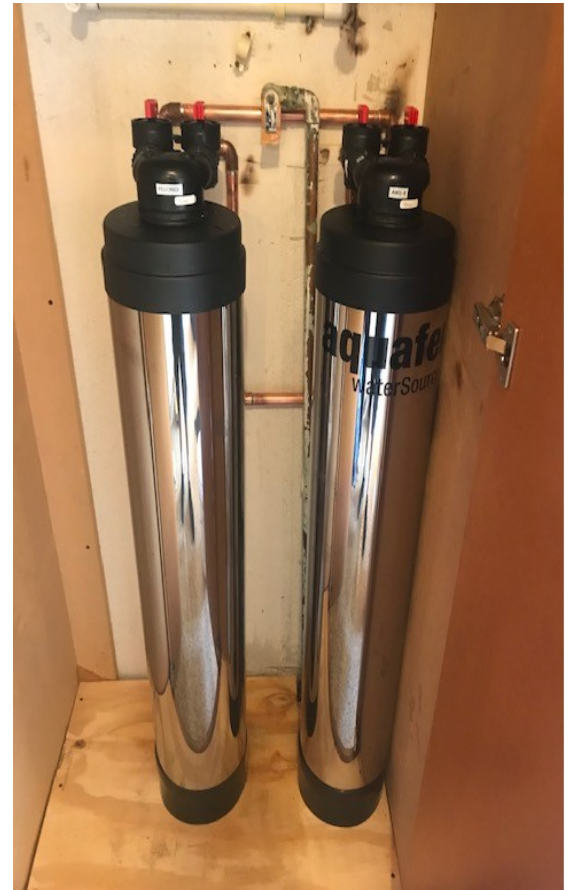
AWS-DHA-9 IN UTILITY CUPBOARD
